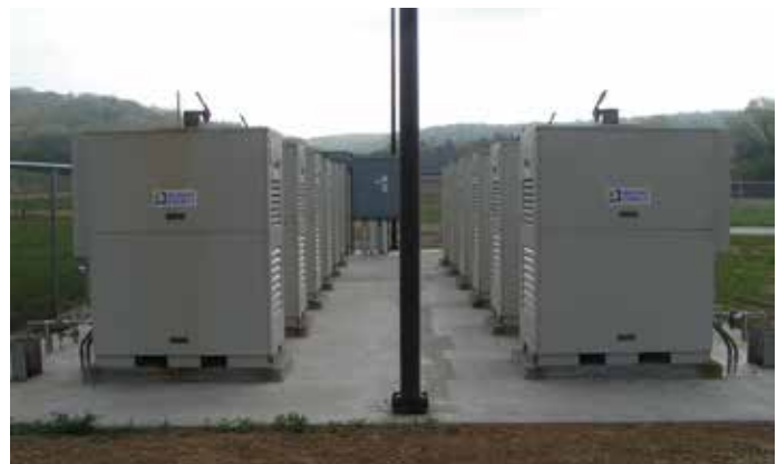
Twenty-four methane-powered Capstone microturbines provide electricity to the Sauk County Landfill in Wisconsin.
