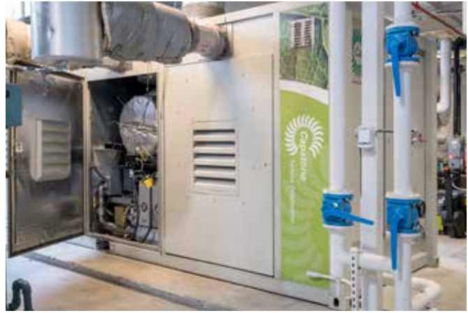
A C1000 microturbine at the VA Medical Center in Ann Arbor, Michigan provides electricity and steam to the 1.1-million-square-foot facility.
