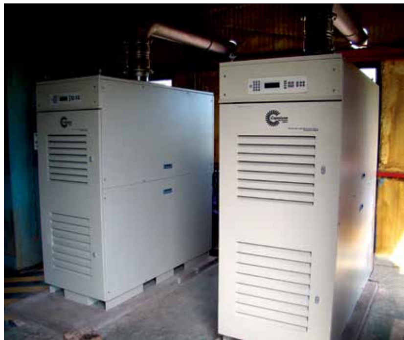
Thirty-five Capstone C65 natural gas-fueled microturbines power compressors at this Bolivian pumping station.
