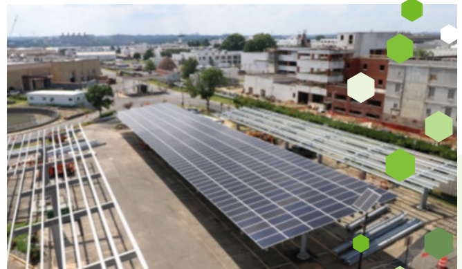
Ameresco's 4.4 MW DC Water Solar PV project
