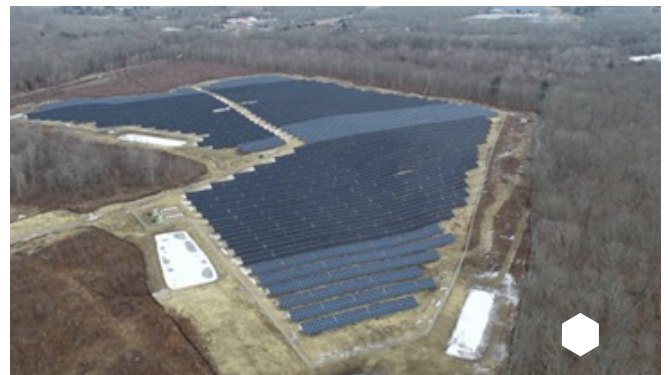
Greenskies Clean Focus' (GCF) 6.1 MW Solar PV project
