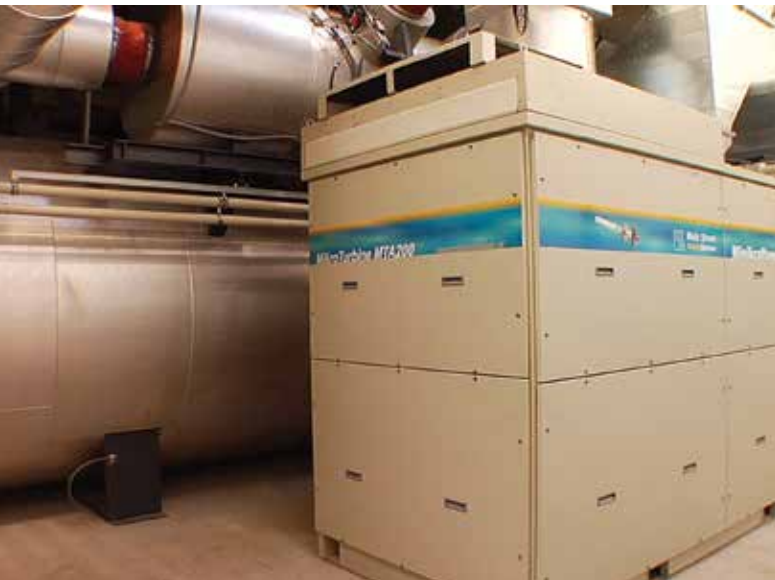
A Capstone C200 microturbine installed in a CCHP application generates electricity for the Machland food manufacturing plant.
