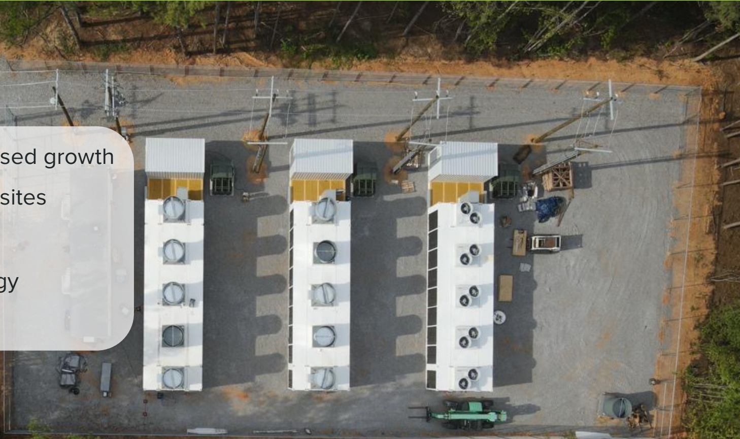
11 MW site in Mississippi
