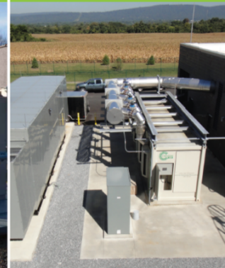
Bank with Data Center
