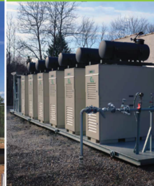
Gas Gathering Facility
