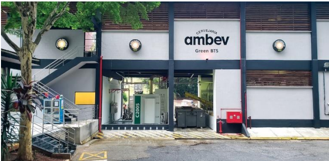
Capstone C200S Microturbine in a CHP Application Generates Clean and Reliable On-site Power for Brewery Giant Ambev in Guarulhos, Brazil.
