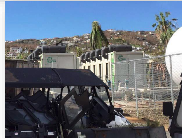
Fully operational Capstone Microturbines on St. Thomas surrounded by debris from Hurricane Irma
