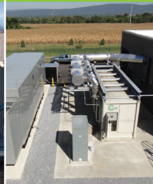
Bank with Data Center
