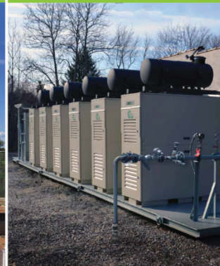
Gas Gathering Facility
