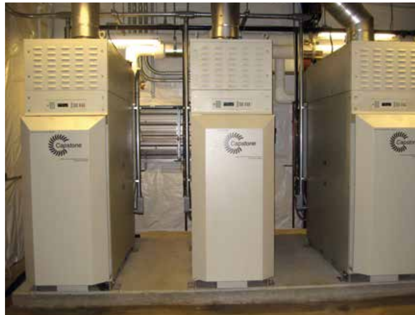
Commissioned in late 2009, the three natural gas C65 ICHP Capstone microturbines produce more than 80 percent of Davidow Hall's electricity and 100 percent of the building's heating and cooling.
