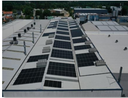
Portugal Photovoltaic Solar Project
