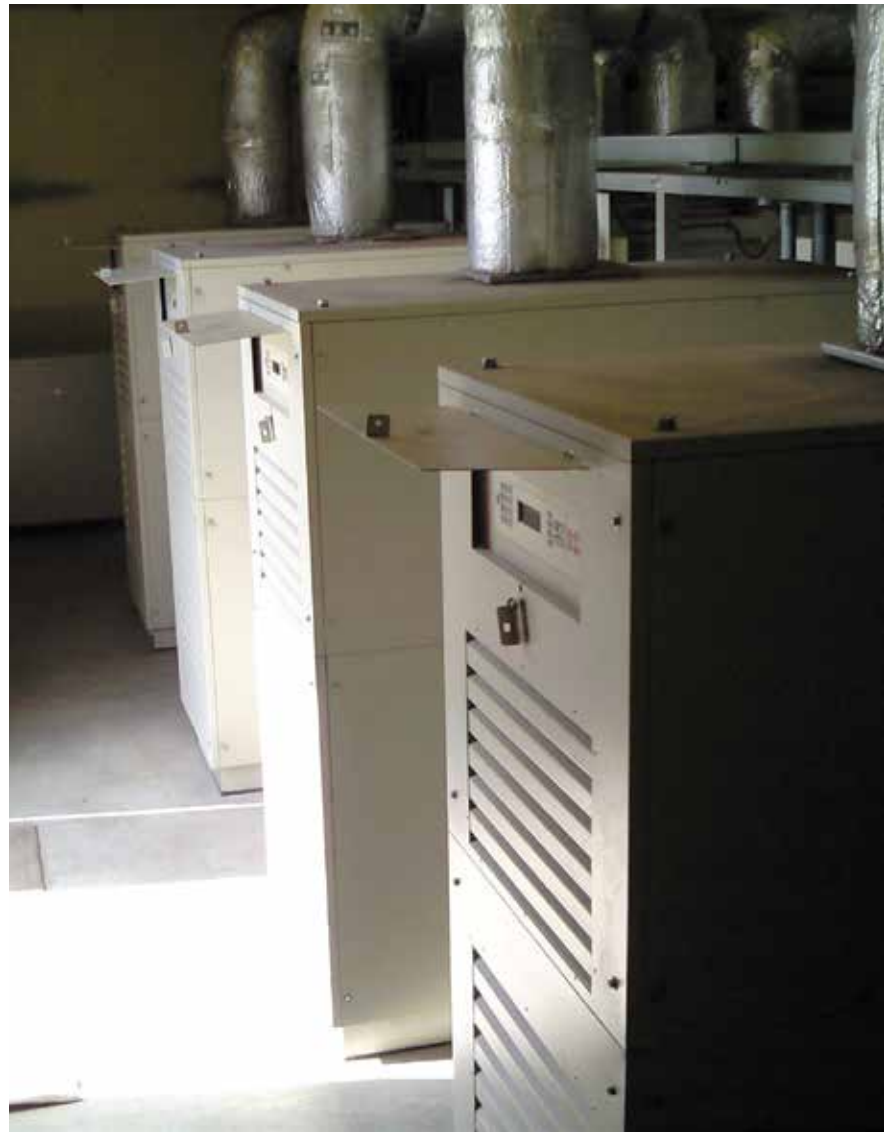
Methane gas fuels four C30 microturbines at a waste-processing center in Japan.
