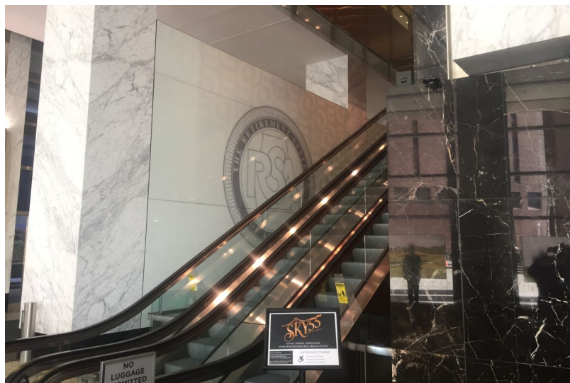
At 55 Water Street, one of the largest office buildings in Manhattan, the gunfire-detection sensors are scattered through the lobby and beside an escalator. PHOTO: CHIP CUTTER/THE WALL STREET JOURNAL
