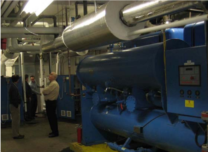
One of two 400-ton gas-fired chiller and heating plants at the Jewish Home and Hospital replaces all-electric chillers. By eliminating peak power rates, comparative operating cost are expected to decline by over half.
