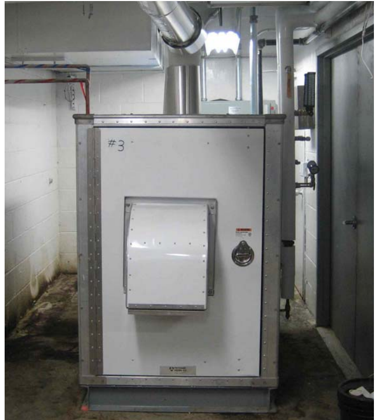
One of three 100-kW Tecogen heating-and-power cogen plants installed at the Jewish Home and Hospital in the Bronx, early in February 2008. This one is tucked into a small, unused alcove.
