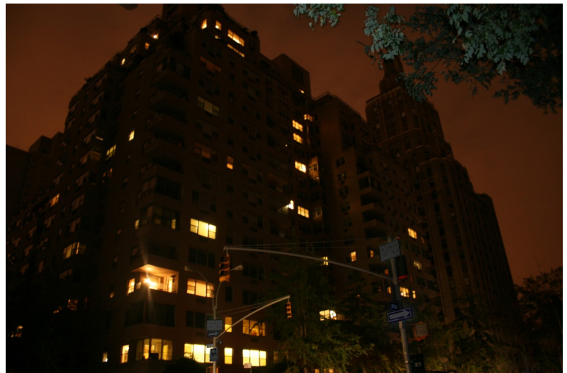
The Brevoort three nights into the Hurricane Sandy blackout with lights shining powered by four Tecogen InVerde CHP units.
