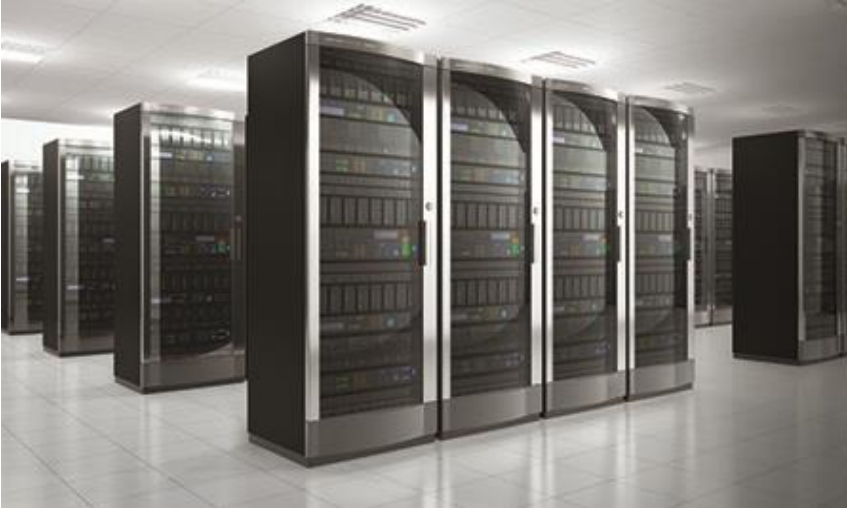
Data Center Optical Fiber
