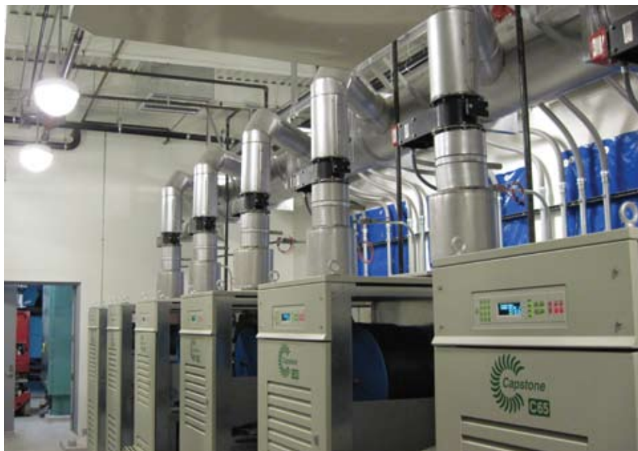
Key components of the US $12.4 million Green Data Center at Syracuse University are 12 patented Capstone Hybrid UPS Microturbines from Capstone Turbine that provide power to the entire facility.
