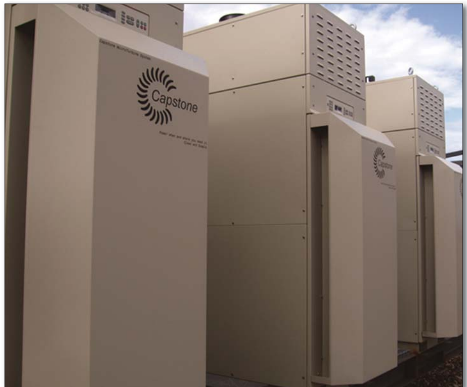
Figure 1: The Four Seasons installed three 65 kW microturbines from Capstone on its roof as part of a CHP project
