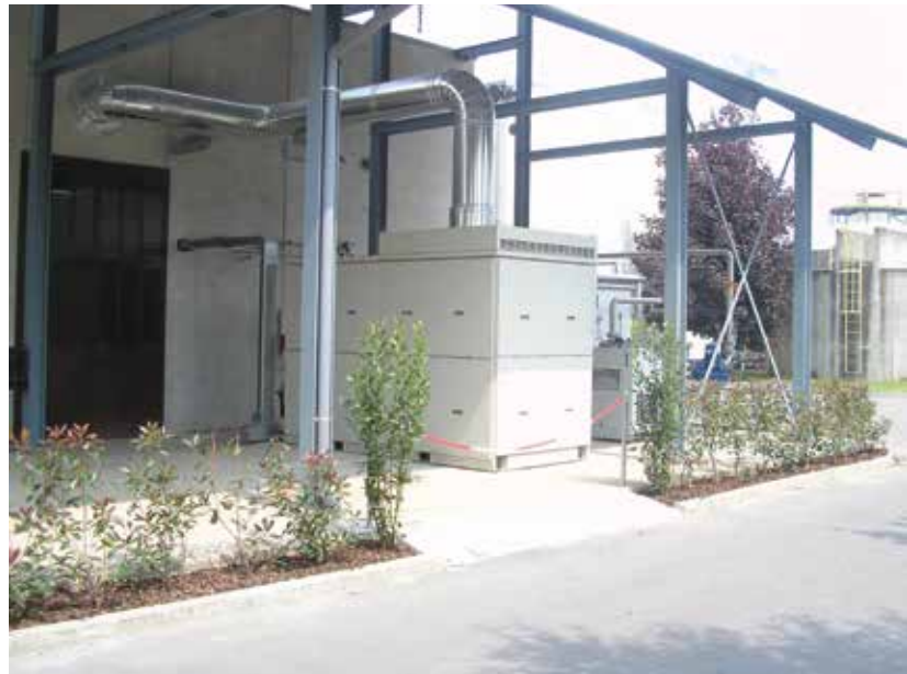
A single Capstone CR200 microturbine fueled by biogas provides all the electrical power needed at the Cossato Spolina Wastewater plant in Italy.
