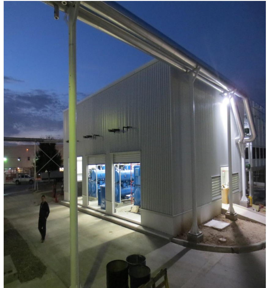
Tecochill chillers keep Mexican factories cool, despite often unreliable grid power.
