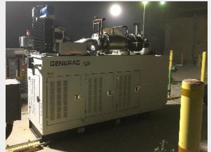
Natural Gas Generator Upfitted with Ultra in Southern California (LA County)
