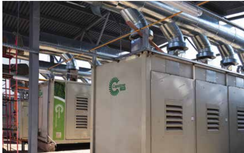
Four natural gas fired Capstone C1000 microturbines operating in a CHP application produce 4MW of clean and reliable power as well as 4.8MW of thermal energy for the Slutsk Cheese Factory.
