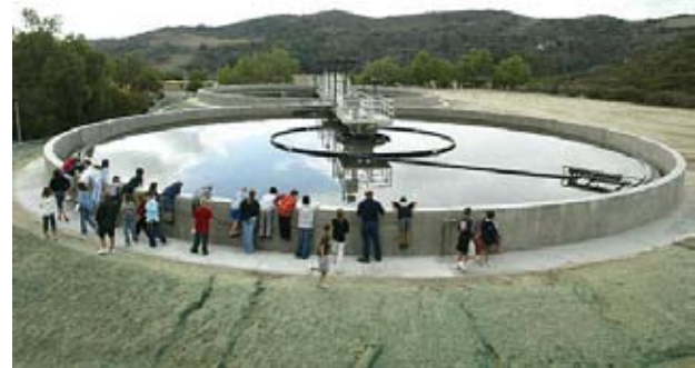
Santa Margarita Water District has a dedication to educating youth about water. Here some school children take a look at a settling pond at the Chiquita facility.
