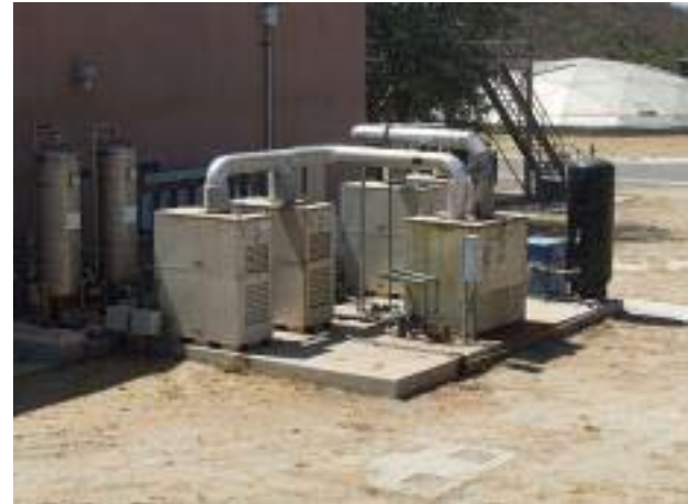
Santa Margarita Water District burns methane for power through the use of these microturbines at their Chiquita Water Reclamation Facility. Using the microturbines saves the district up to $8,000 a month on power.
