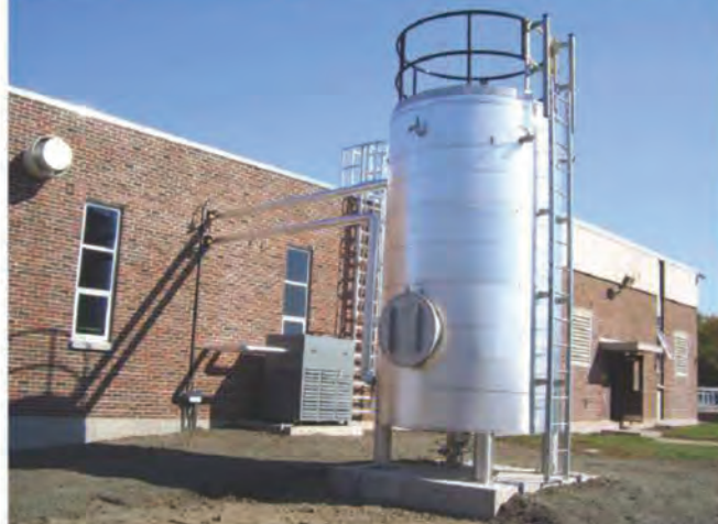
The gas treatment skid (Unison) removes contaminants like organic siloxanes from the biogas to protect the microturbines. The hydrogen sulfide removal vessel is located outdoors next to the plant.
