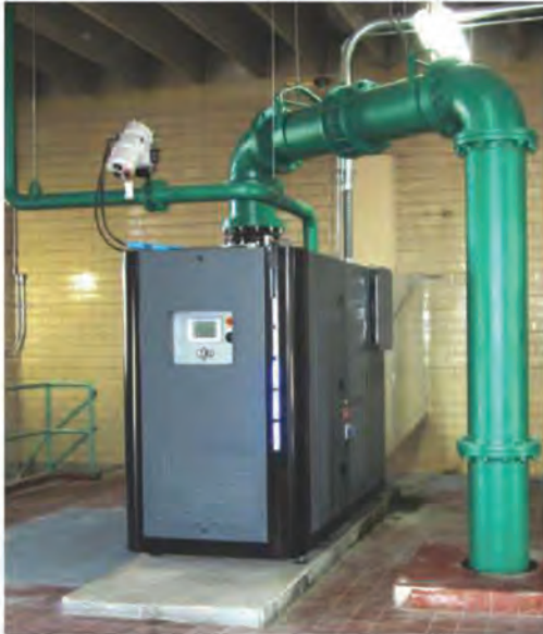
Turblex blowers have improved aeration at the Wausau Wastewater Treatment Plant while also reducing energy needs.
