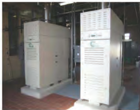
Two Capstone 65 kW microturbines will help the plant avoid buying nearly 1 million kWh and 77,000 therms of natural gas from the local utility every year.
