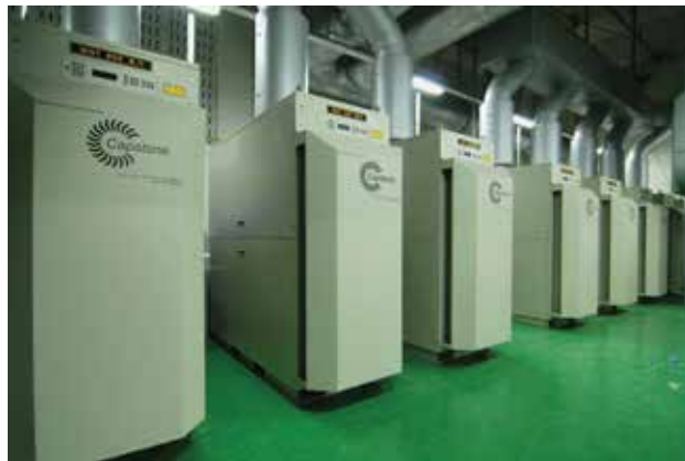
Ten C65 microturbines provide electricity and heating to a 44,520 square-meter (479,209 square-feet) apartment complex in South Korea.
