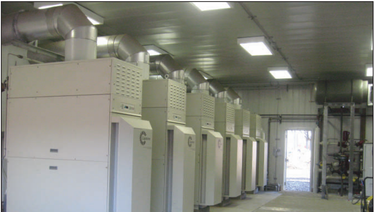
Basic Systems Inc. designed the expansion of this gas storage facility in remote north central Pennsylvania, U.S.A. Six Capstone C65 microturbines were initially installed to provide the additional power required for the expansion.
