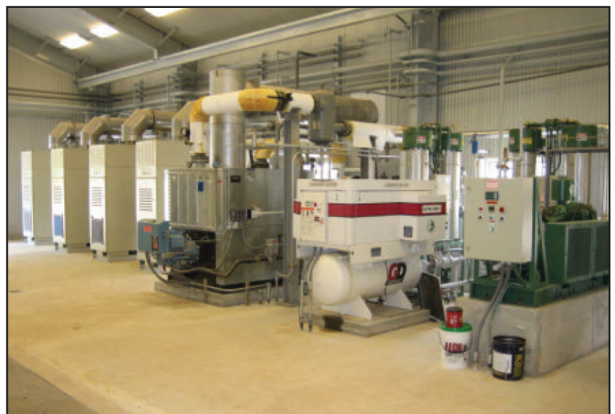
Four of nine compact Capstone C65-ICHP microturbines with exhaust heat recovery, shown in a facility designed by Basic Systems Inc. The nine microturbines provide all of the electrical power for a new compressor station at a remote gas storage site.
