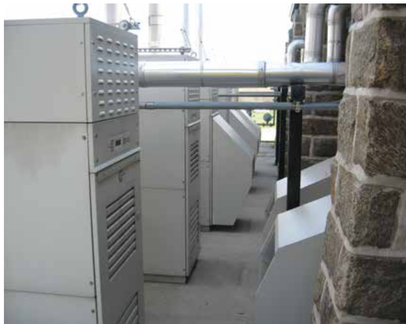
Capstone microturbines generate electricity and heating at Masonic Village, a 1,400-acre complex serving more than 1,700 residents since 1910.
