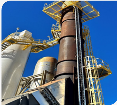
Plenum Breach for Ports
