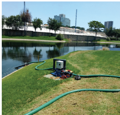
Installation of the Moleaer nanobubble generator does not require submersion into the pond.
