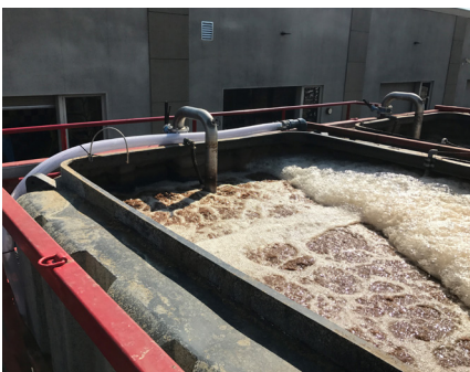
Picture 2: MBR aeration tank
