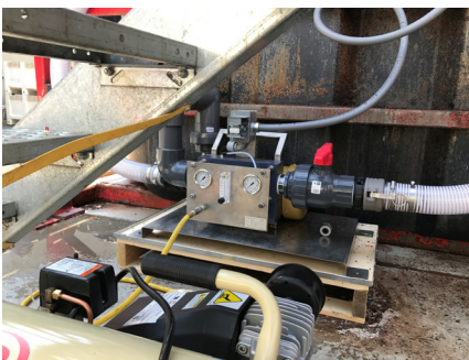
Picture 1: Moleaer XTB retrofitted outside MBR tank
