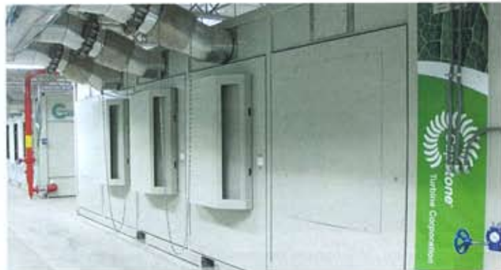
Photos courtesy of Flex Energy and E-finity Corp.
