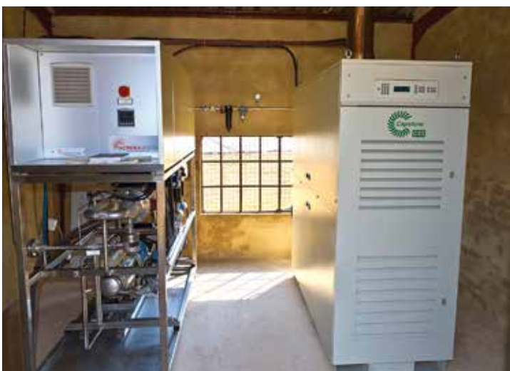
A digester gas-fueled Capstone CR65 microturbine provides power to Swineline Farm in South Africa.
