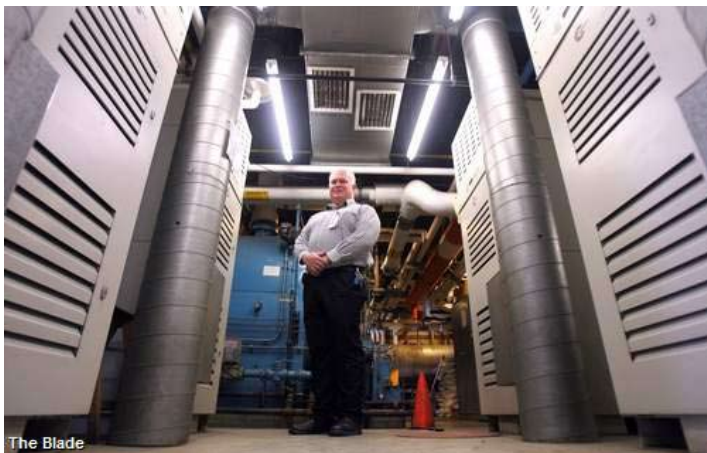
Paul Bernard, physical plant manager, estimates the turbines save the museum about $500,000 in utilities costs annually. (THE BLADE/AMY E. VOIGT)
