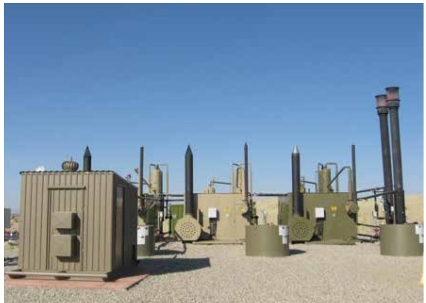
The remote Jonah Field wellsite uses a Capstone C30 microturbine to generate electricity to run the site's pumps.
