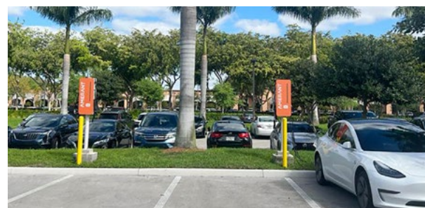
Charging stations at Miramar Operations Center.
