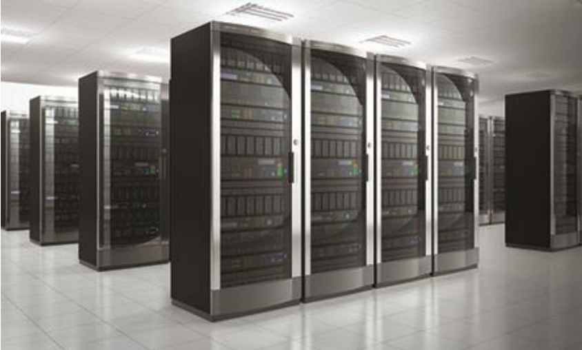
Data Center Optical Fiber
