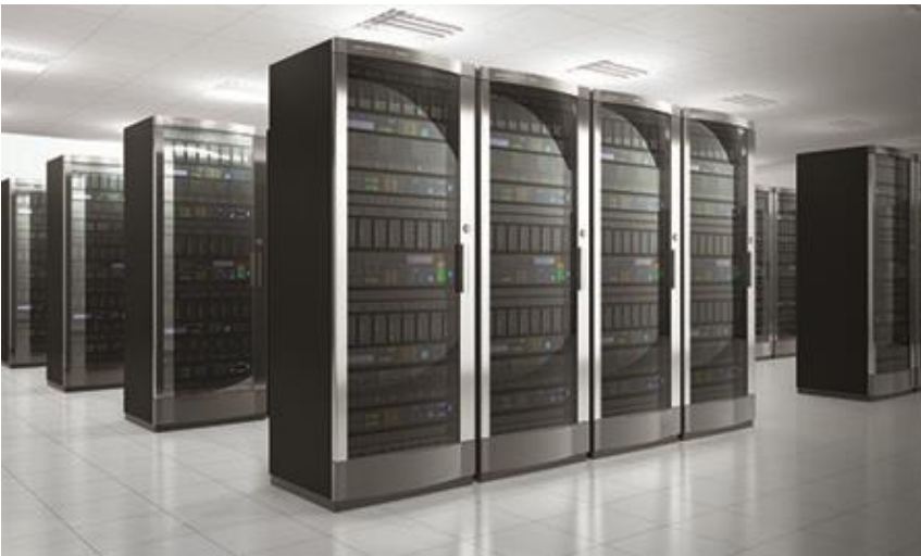
Data Center Optical Fiber
