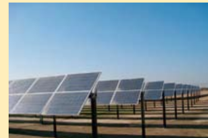
The North Face ® brand’s distribution center in Visalia, California, utilizes solar panels to power 25% of the facility’s energy needs.
