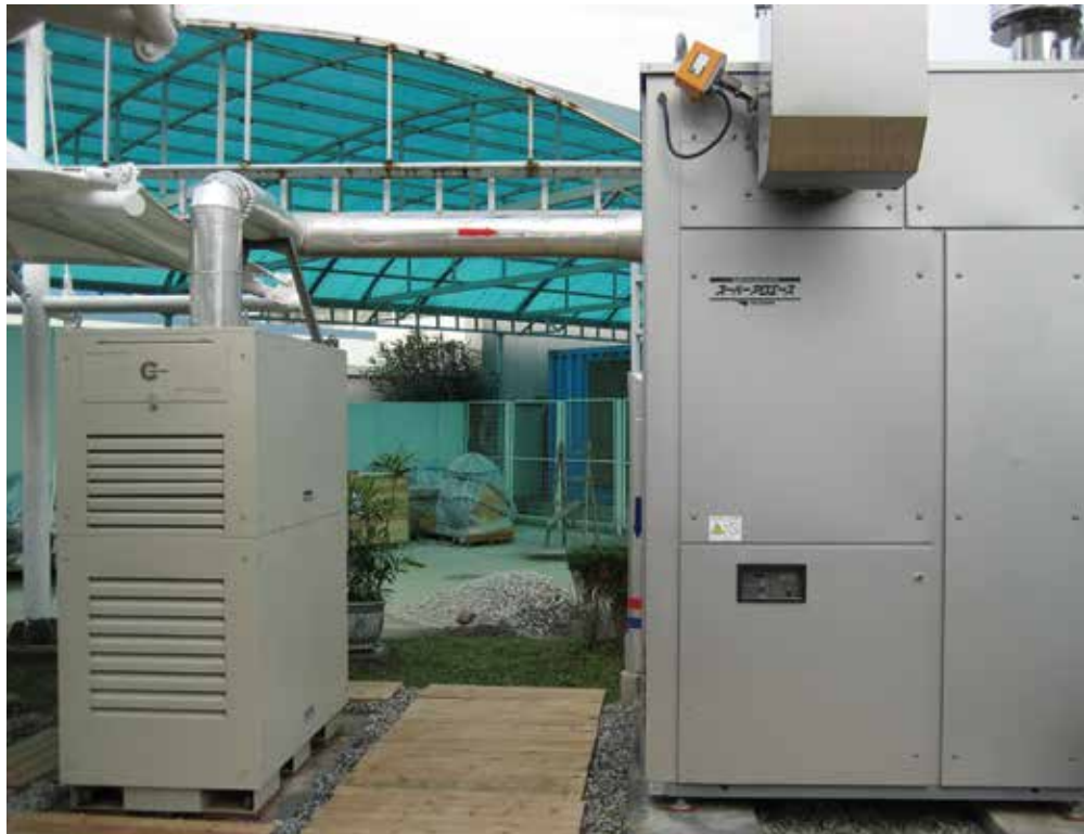
A Capstone C30 microturbine providing electricity and heating, is installed at Shanghai Aerospace Energy in Peoples Republic of China.
