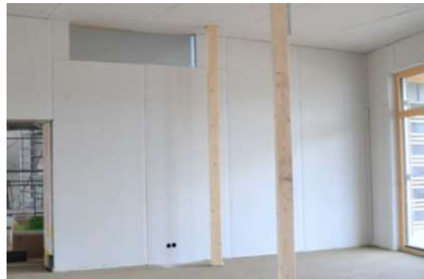
Fermacell fiber gypsum - interior of Kindergarten in Brittany, France
