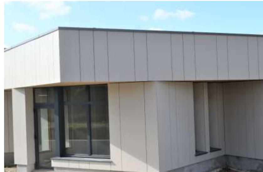
HardiePanel fiber cement - exterior of Kindergarten in Brittany, France
