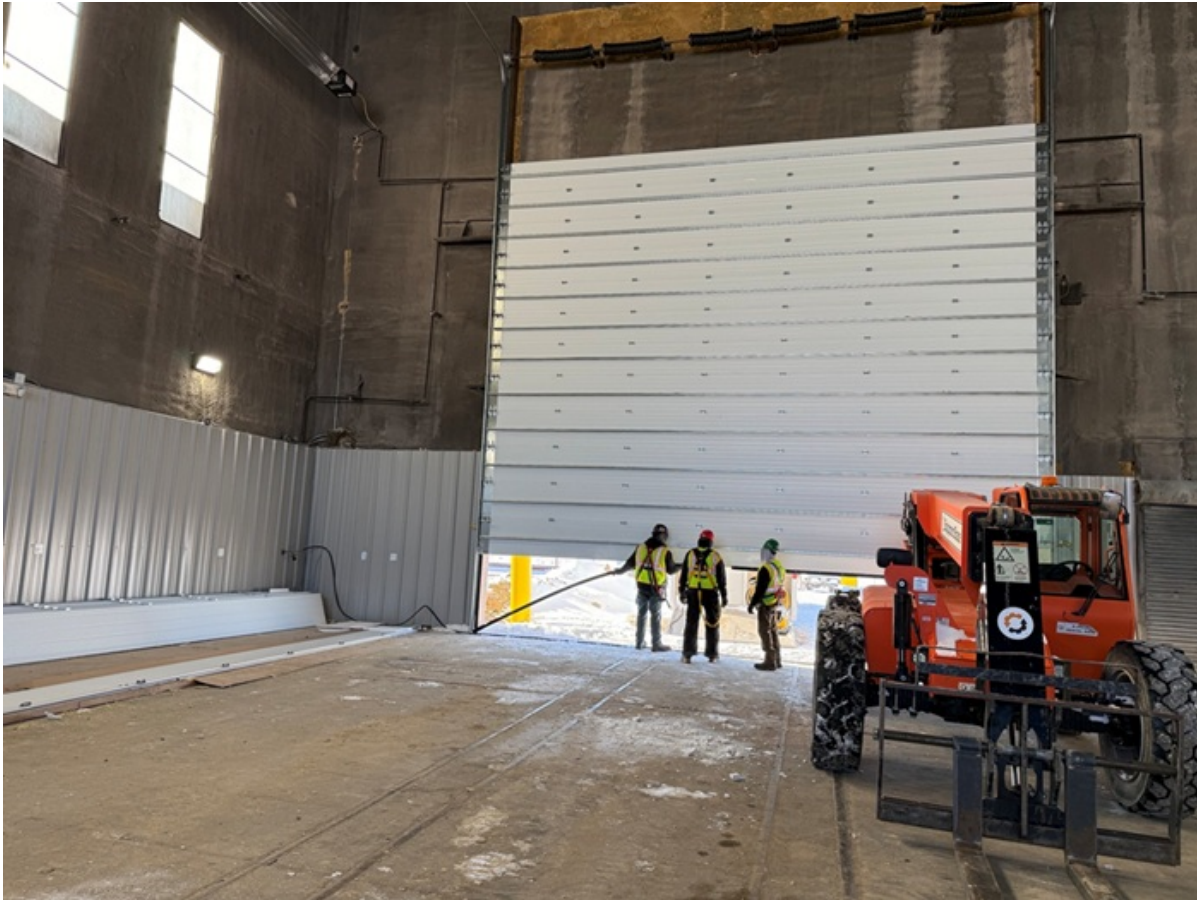
Interior of conventional mine "lube bay" that is being updated so it can be used for maintenance activities. Total square footage is 4,000.
